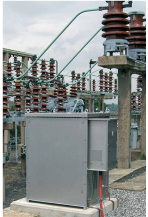
NGR constructed from 304 stainless steel
